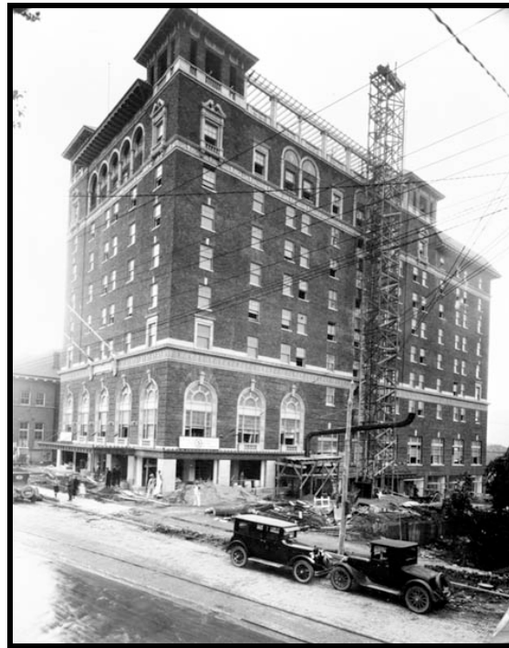
Figure 7: George Vanderbilt Hotel, under construction (E.M. Ball Collection, Ramsey Library Special Collections, UNCA, N1832).
